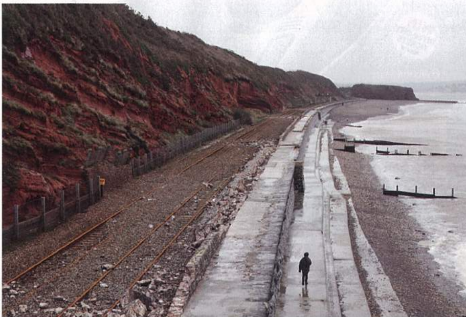
The damage caused at Dawlish further east, between Rockstone Bridge and Langstone Rock, was more superficial, with the wall separating the pedestrian walkway and the tracks now strewn over the railway. This was the view on February 5. ANTONY CHRISTIE.
